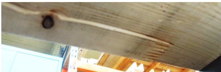
Figure B.31: Finger joints damage of test specimen G02
