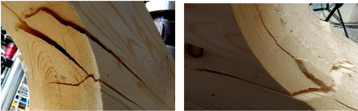
Figure B.19: Fully spread cracks on the upper left (left) and lower right (right) opening edge of specimen D03
