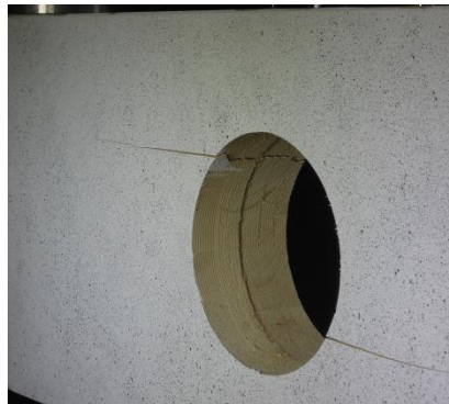
Figure B.3: Tensile stress perpendicular to the grain on the upper left and lower right opening edge of the specimen B02
