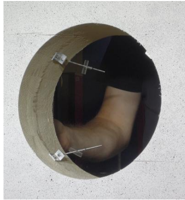
Figure B.13: Tensile stress perpendicular to the grain cracks on the upper left and lower right opening edge of specimen D01
