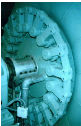
Figure 1-16: Operating ring and attached links to operate the guide vanes (Source: [3a])
