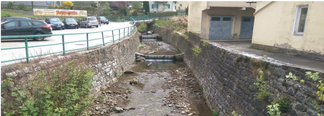
Figure 4-6: River bank reconstruction and weirs built for flood control in St. Getraud (Austria)
