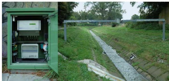
Figure 4-7: water level measuring station
