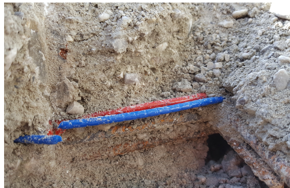
(f) Exposure of fibre-optic cables after the test.
