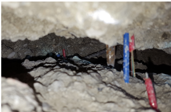
(e) Severed fibre-optic cables due to failure.
