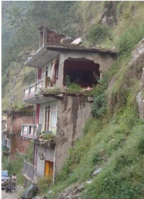
Figure 70 Destroyed house in Kodari ( 27^{\circ}58'17.12''\text{N} , 85^{\circ}57'41.78''\text{E} ). Before (left) and after (right) the monsoon (© Ziselsberger).
