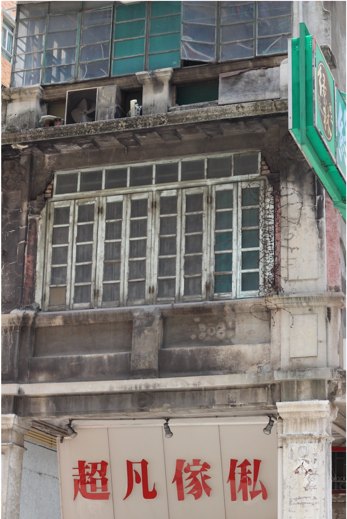
Abb. 262: Facades are mildew and getting dark caused by the Humidity
