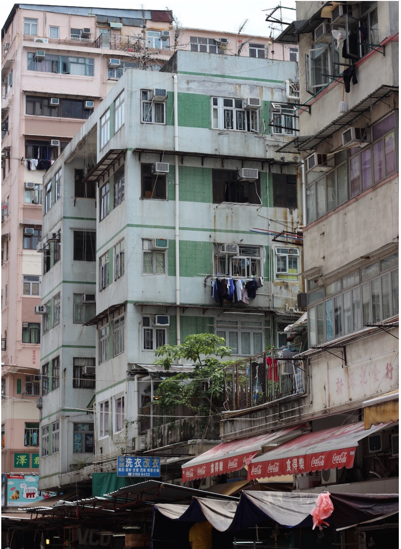
Abb. 263: Because the Buildings do not really have a sealing, the Humidity can slowly destroy the Building
