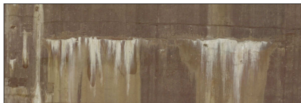
Figure 6-3: Rectified detail image of the defect in block 16 of the Drossen dam, 2 mm/px
