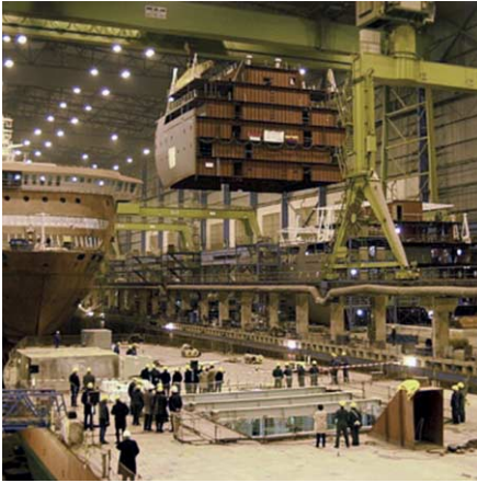
FIG. 69 A 6-storey high prefabricated part of the ship is craned to the main hull. [source: www.meyerwerft.de]
