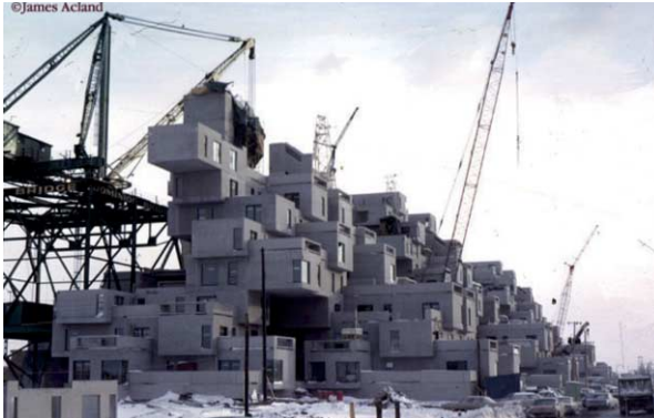
FIG. 31 Moshe Safdie's Habitat for Montréal under construction in 1967. [source: Fine Arts Image Library, University of Toronto, photographer James Acland]
