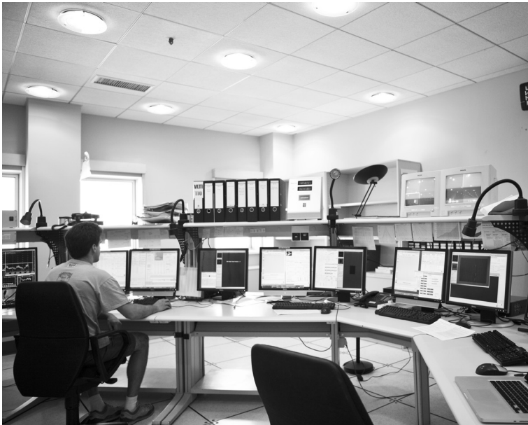
034 Control Room during daytime
