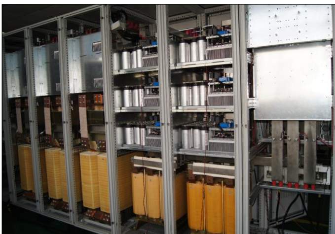
Figure 6-2; Back of the power amplifier (Remove cover plates)
