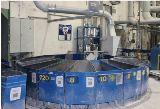
Figure 3-6: Carousel for dosing bulk solids for cored wire
