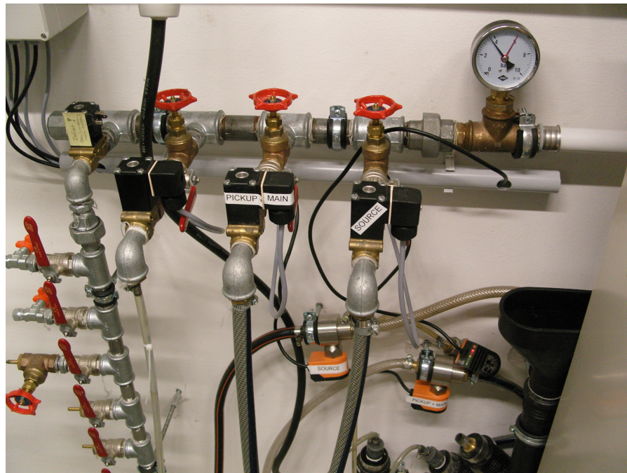
Figure A.10.: Connections of the cooling circuit. The black solenoid valves can be controlled via the control panel. The orange flow monitors in the return are adjustable via a potentiometer.
