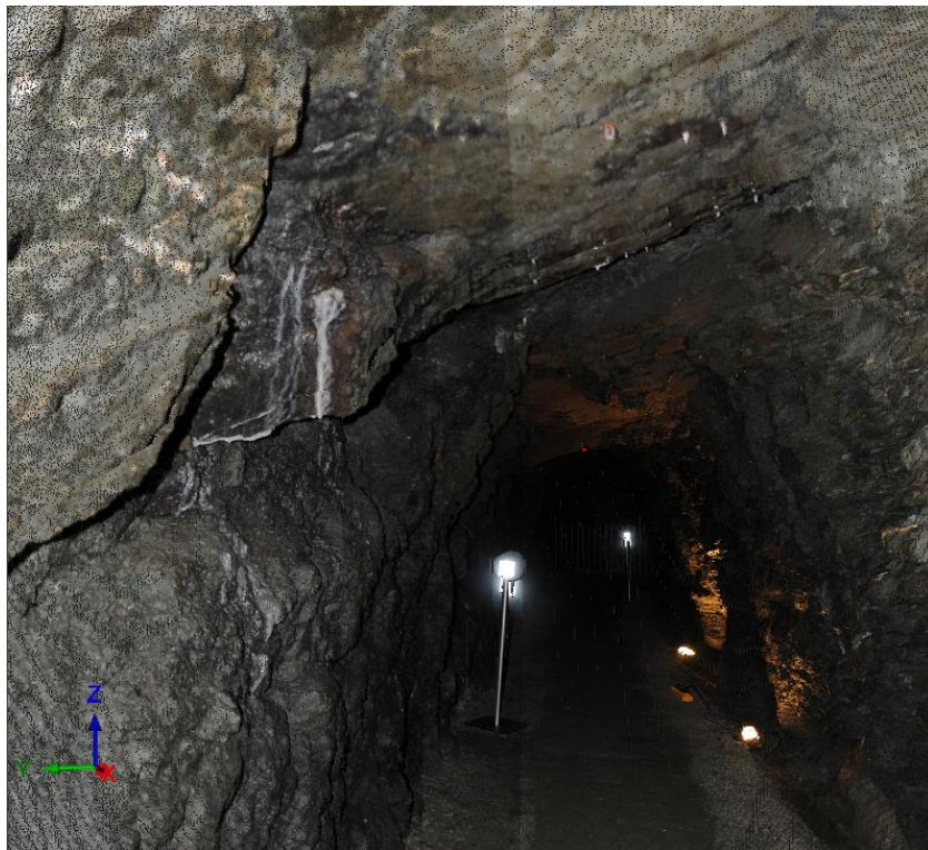
Figure 4.6: Screenshot of 3D LiDAR point cloud model: overbreaks due to fault zone, view to the east (After Liu and Kieffer, 2012)
