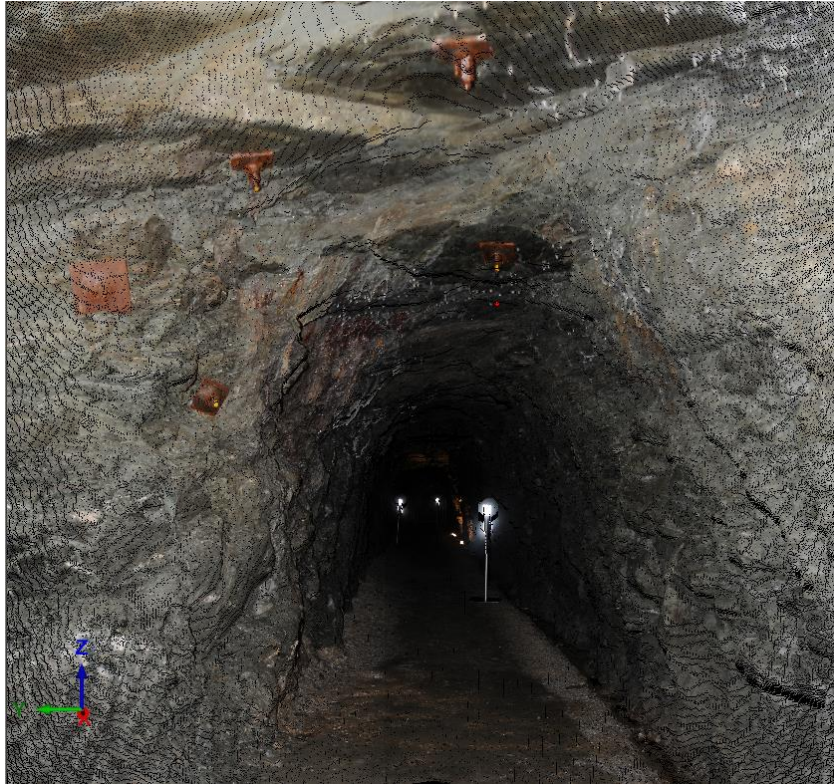
Figure 4.5: Screenshot of 3D LiDAR point cloud model: rock bolts stabilising schistosity and joints, view to the east (After Liu and Kieffer, 2012)
