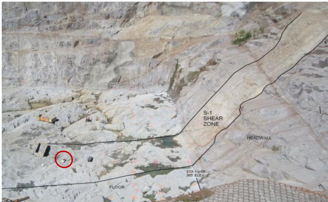
Fig. 5-8: Photograph, looking North from the left cut slope, showing S1 in the headwall and the floor of the spillway during phase II excavation. The red circle indicates two cars for scale, (U.S. Army, Corps of Engineers, 2012).
