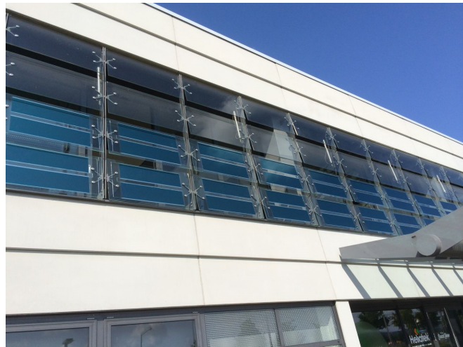
Figure 5.4: Building integrated organic photovoltaic (BIOPV) [39]
