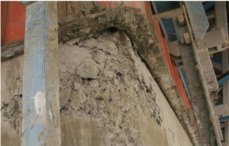
Fig. 4.12 Defective corner with slipform 53
