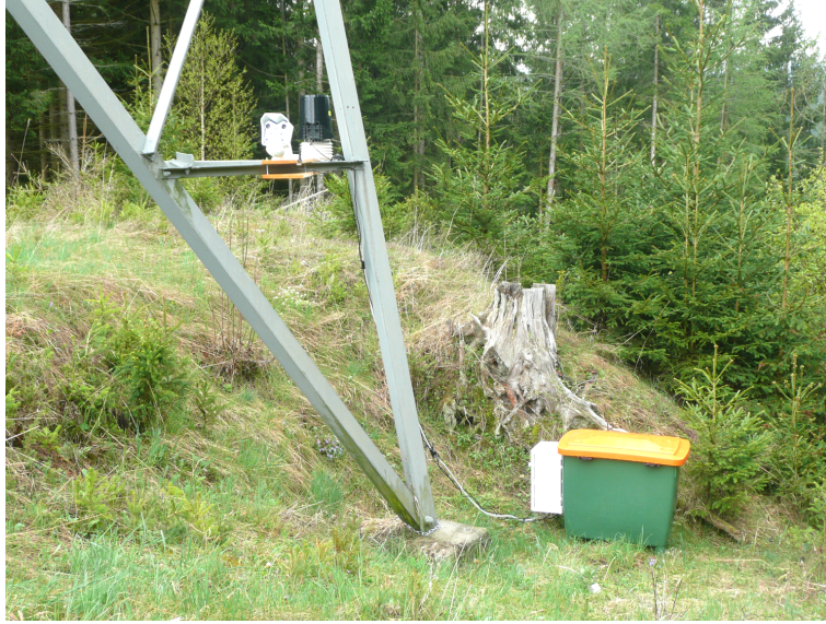
Figure 8.5: Overview of the base station, containing weather camera and meteorological sensors on the transmission tower and a battery container (green/orange).
