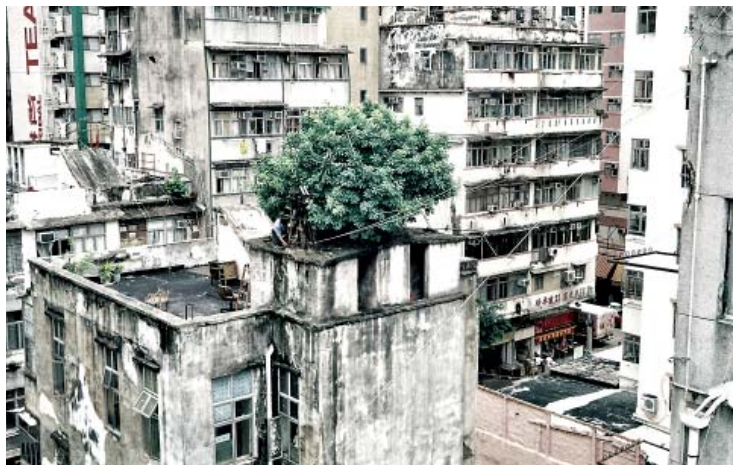
016 Fig tree on rooftop
