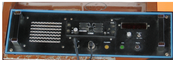
(b) Airport tower transceiver.
