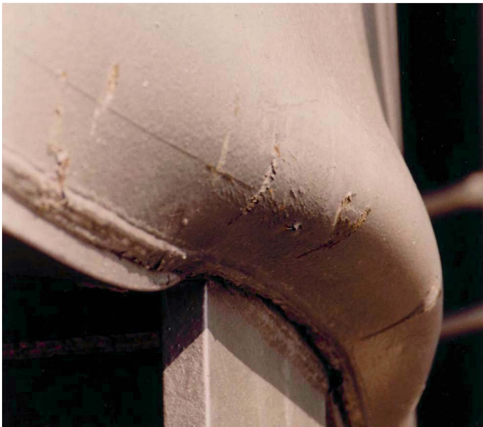
Figure 1.4 Elephant's foot buckling above a column support (Guggenberger)
