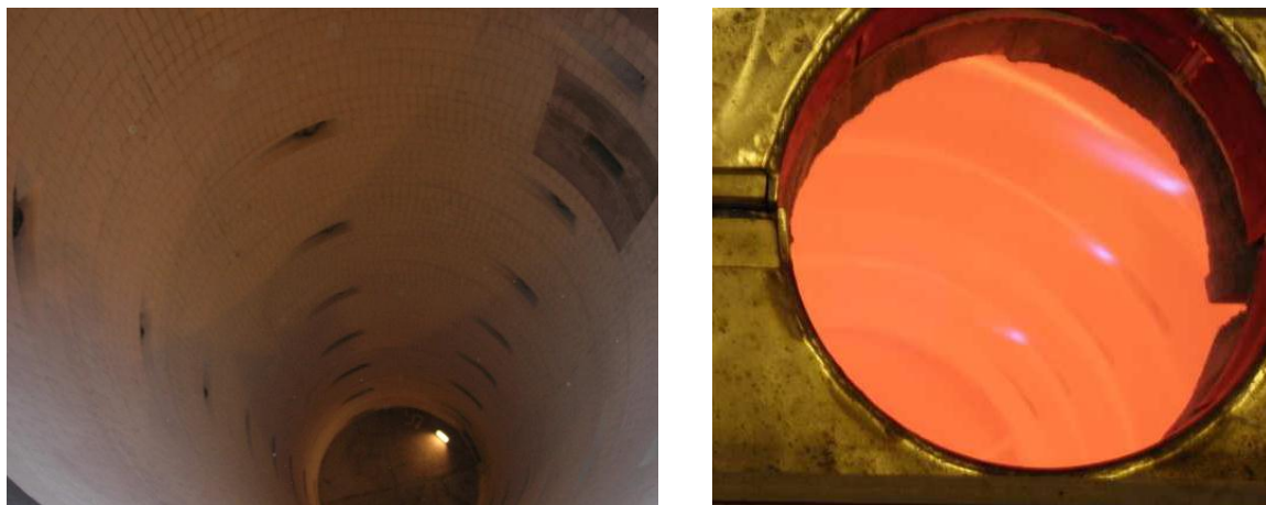
Fig. 4.13: Gas-fired heat-treatment furnace [Andritz-Maerz 2009, p.3]
