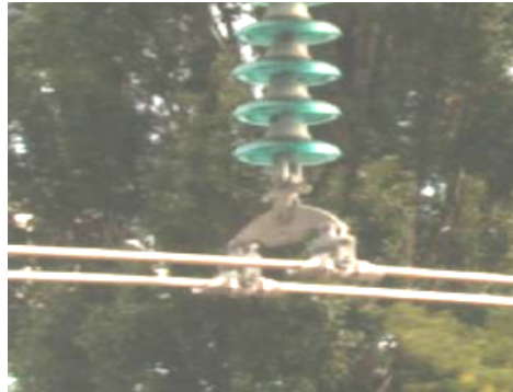
Figure 6.25: Insulator plus conductor without corona ring
