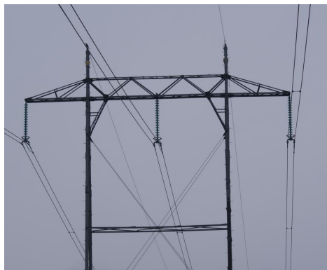
Figure 4.1: Affected tower of Statnett SF
