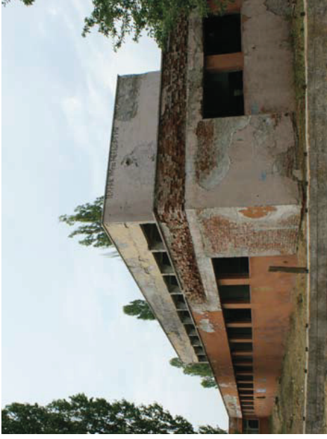
Photos taken from Botumetz reflect a ghost-like atmosphere. After being polluted regularly for almost 5 decades the neighbouring villages experience decline
