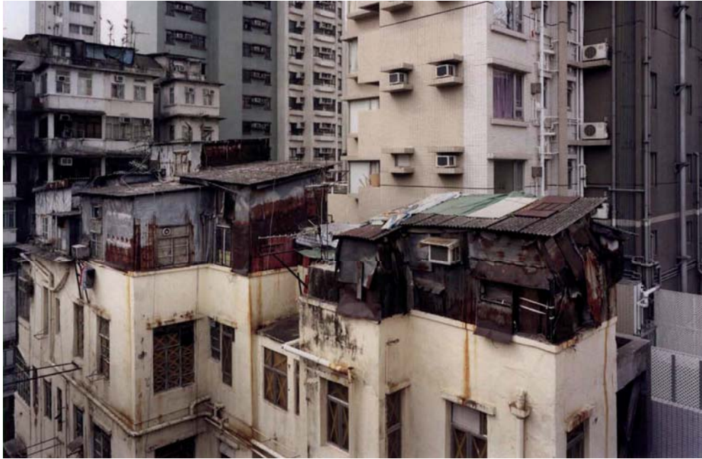
Abb. 4.15 Illegale Dachaufbauten in Sham Shui Po, Photo
