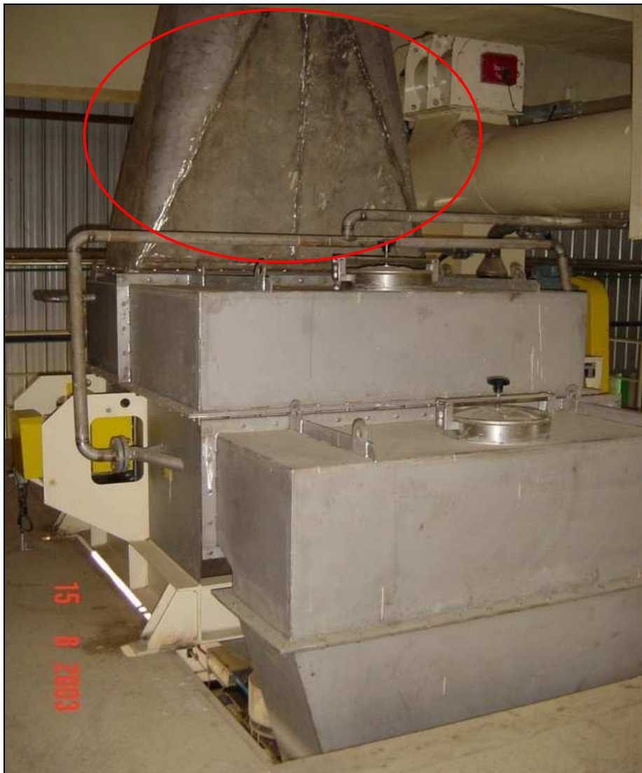
Picture 1: Installed chip washer with inlet channel [Andritz internal]
