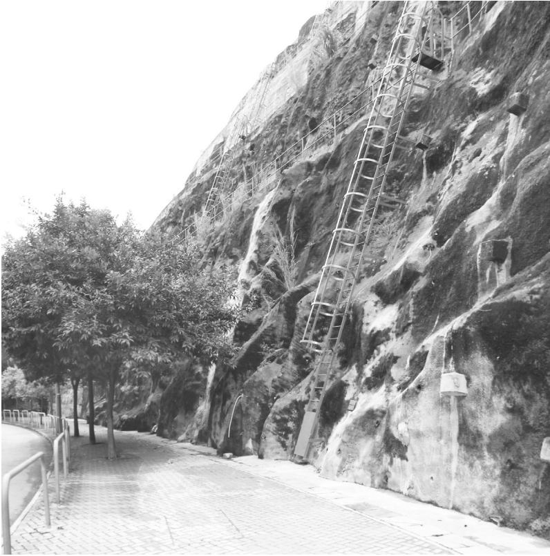
side walk with trees for shading, wheel holes and inspection ladder on shotcrete 'wall'
