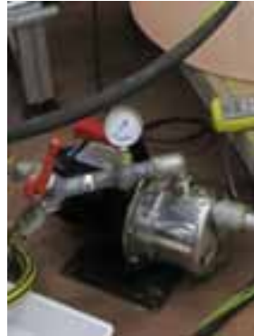
Figure 13: Feed water pump
