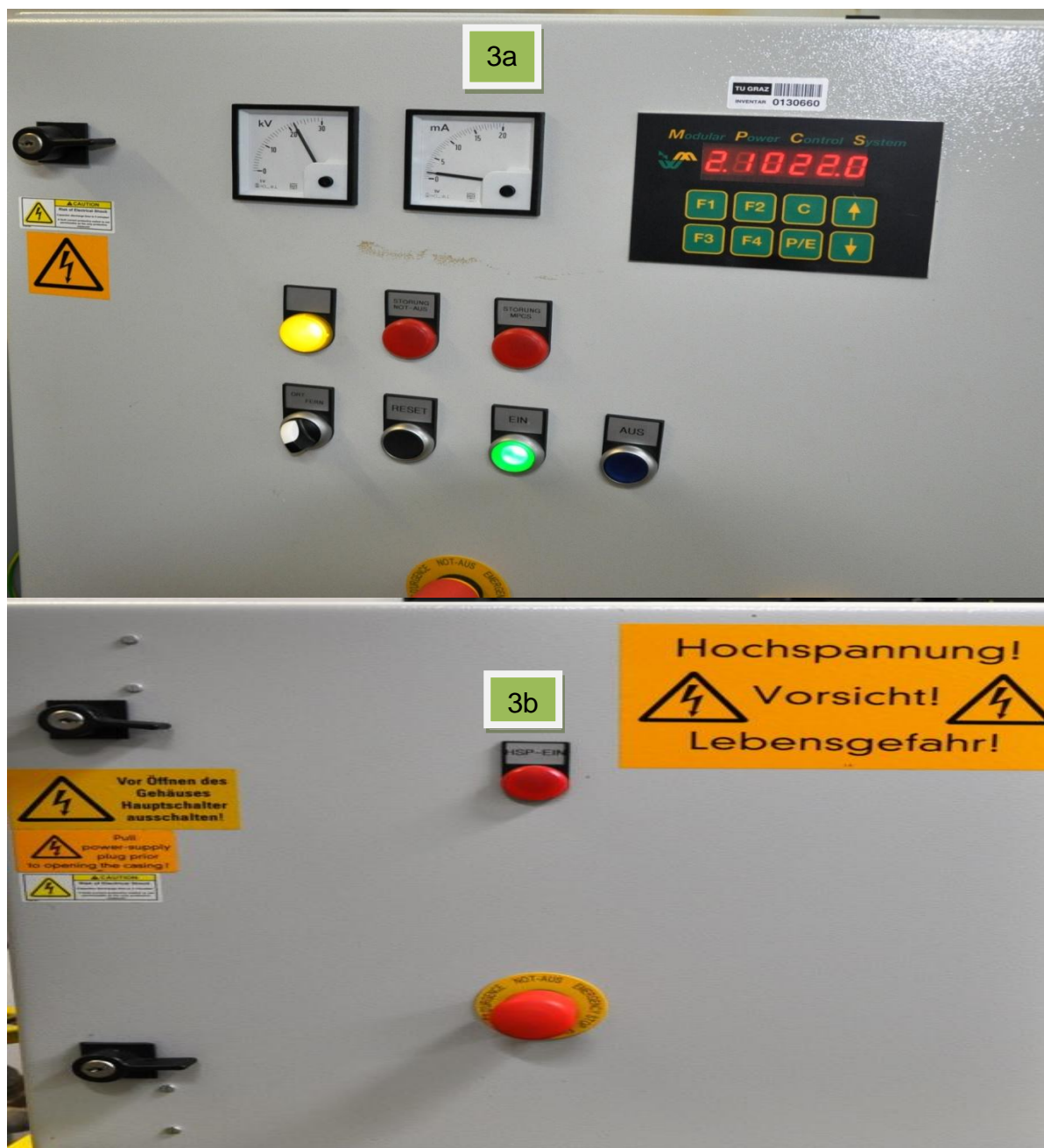
Figure 3: High voltage electrical control panel and DC power supply 3a and 3b respectively used for energizing the wet electrostatic precipitator
