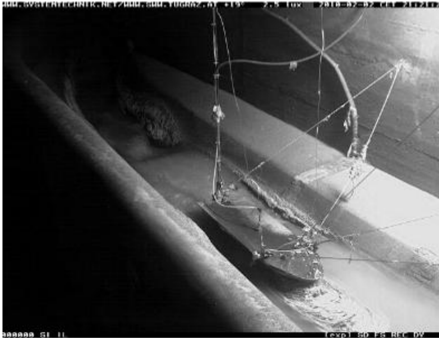
Figure 6-3: View of the overflow chamber and floating pontoon (remote shot from the installed camera, 2010-02-02)
