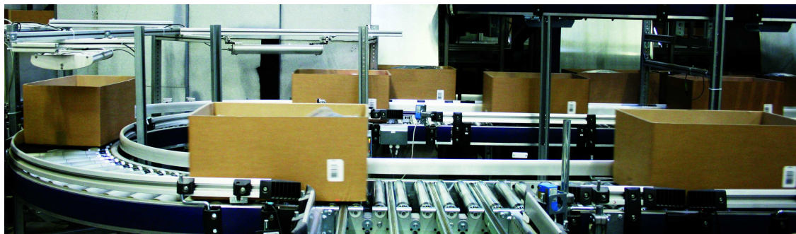
Figure 4.14: RFID readpoints installed on a motorized conveyor belt. The two antennas mounted above the conveyor belt are aligned such that the energy transfer to the tag is maximized. Due to the similar orientation and close spacing, both readpoints show a considerable correlation with respect to the detected RFID tags. Image courtesy of Enso Detego GmbH, 2013.
