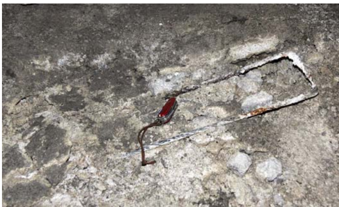
Figure 2 – Concrete heavily damaged by thaumasite form of sulphate attack (TSA).
