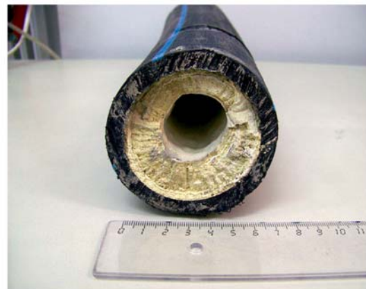
Fig. 1. Drainage tube from the Koralm tunnel with calcite sinter
