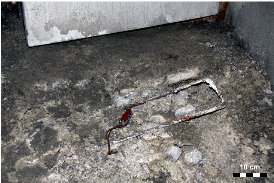
Figure 2. Concrete heavily damaged by thaumasite form of sulfate attack (TSA).
