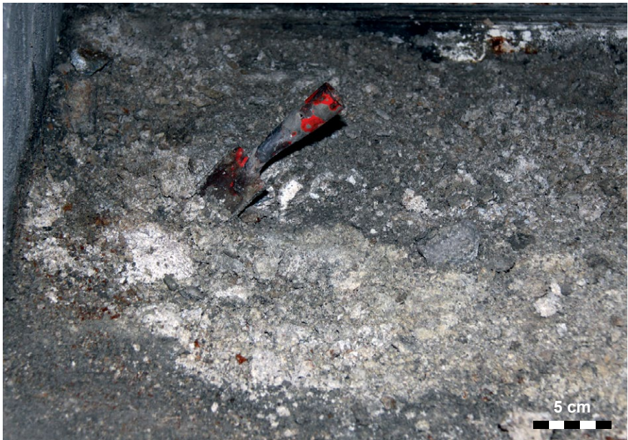
Figure 1: Completely disintegrated concrete found in a ventilation tube of a highway tunnel. The side drainage tube underneath this area is not working properly and water is leaking into the concrete. White mushy material has no cohesion and is sampled by a garden shovel. The mineralogical composition and the corresponding expressed interstitial solution are referred to sample HW_IS01 in Tables 1 to 3 in the following section 3.2. and in the appendix.
