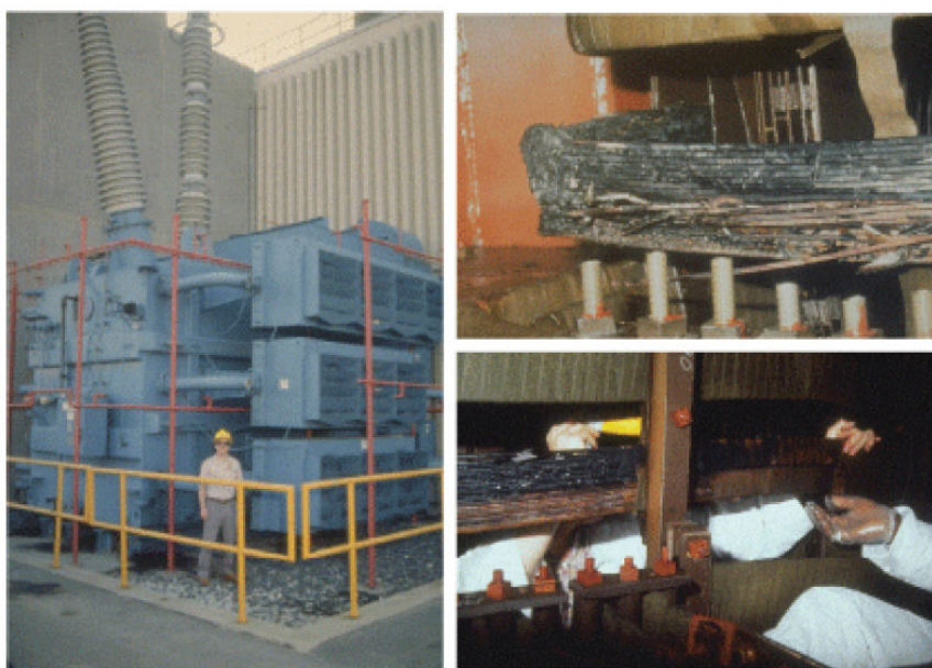
Figure 2.11: Permanent damage to the Salem New Jersey Nuclear Plant GSU Transformer caused by a geomagnetic storm occurred on March 13, 1989. Photos courtesy of PSE&G. The picture was taken from http://science.nasa.gov .
