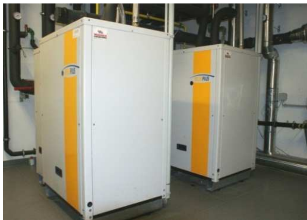
Figure 2-5: Photo of the installed gas-fired AHP units in Graz (Rieberer and Moser, 2011)
