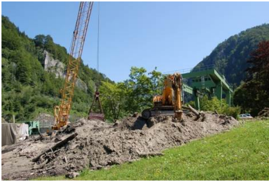
Figure 8.3: Removed sediment from the turbine inlets in July 2009
