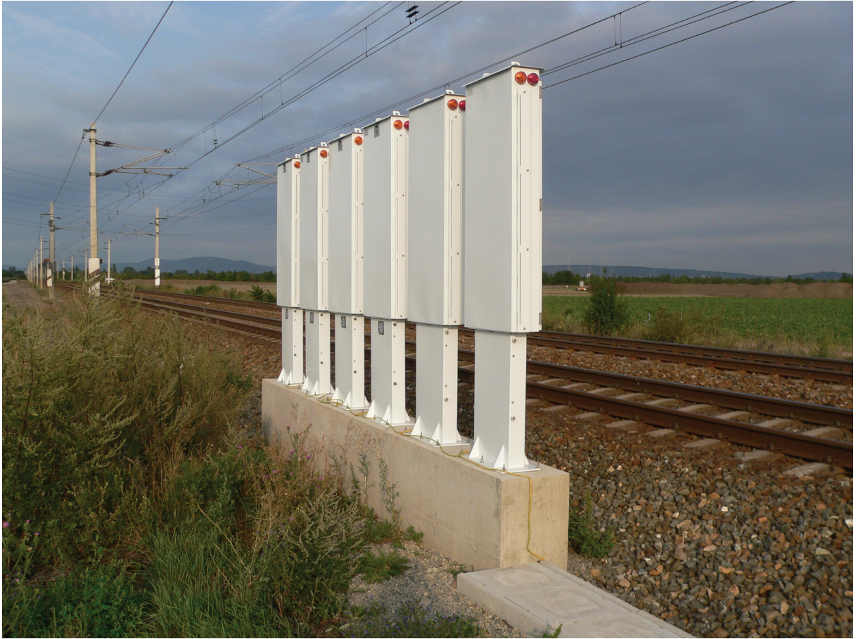
Fig. 15. The monitoring system near Vienna consisting of six daisy chained portals.
