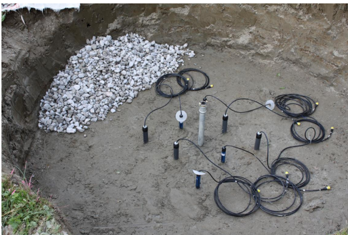
c) Installed air injection pipe and measuring devices; beginning of back filling with coarse gravel.
