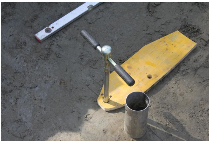
b) Secondary pipe for filter installation; boring of holes for the TDR-probes and tensiometers.
