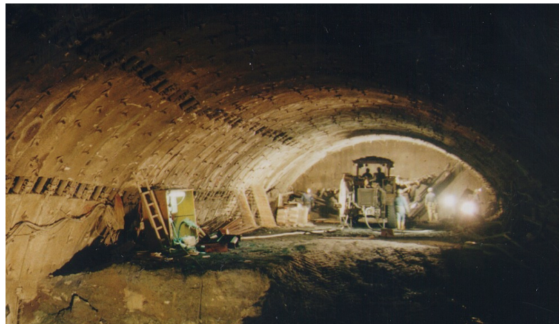
Figure 17. Top heading with four rows of installed yielding elements, Galgenbergtunnel, Haberlstörung (courtesy of Prof. Wulf Schubert)
