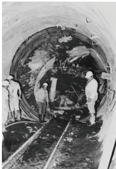
Figure 15. Excavation of the remains of the TBM, Yacambu Tunnel, Venezuela (taken from Hoek, 2009)
