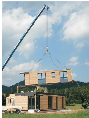
Figure 2-7: a.) Composition of cross-laminated panels b.) On-site erection of a house built using the massive panel system.
