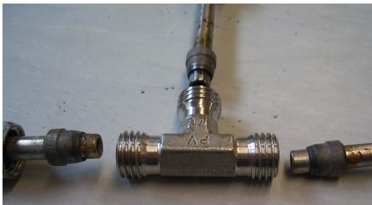
Fig. 6 - 17 Corroded filter unit fittings as source of leakage
