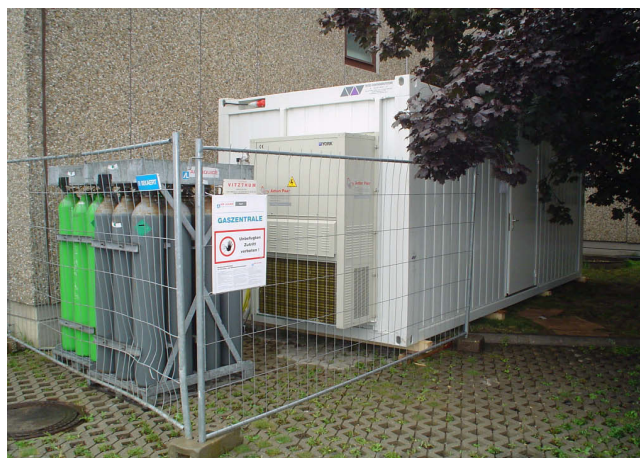
Fig. 6 - 14 Container with argon gas bundles in front of the waste water treatment building
