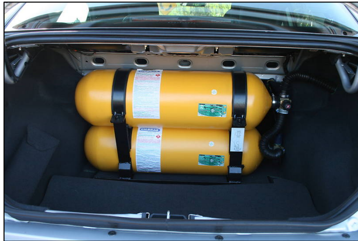
Figure 16: CNG tanks installed in the trunk 179
