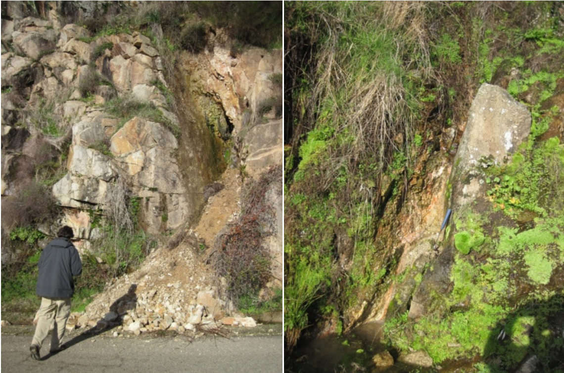
Figure 6.24 – Strong weathering observed along wet discontinuity planes.
