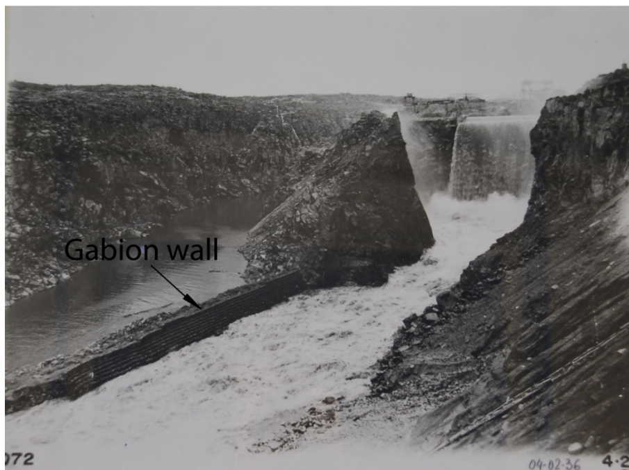
Figure 4.10 – Detail of the spillway after first phase of the fourth scour event in 04/02/1936 (Iberdrola S.A.)
