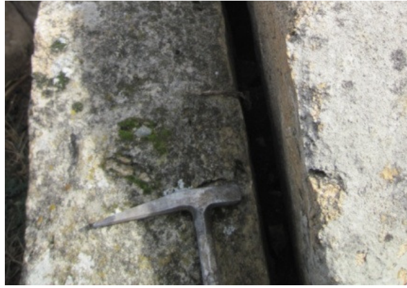
Figure 6.26 – Joint aperture in unstable areas
