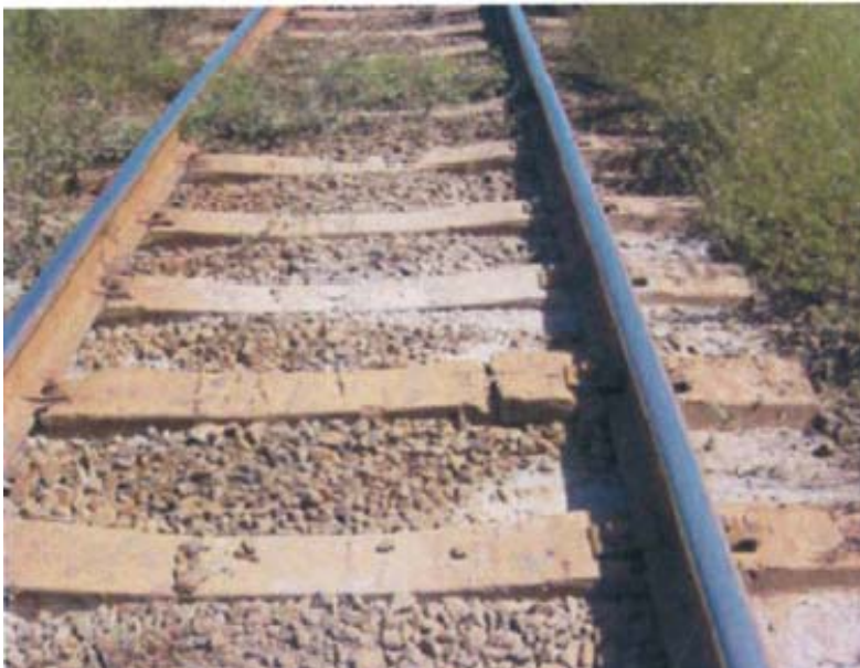
Picture 18: Broken sleeper in fouled ballast
