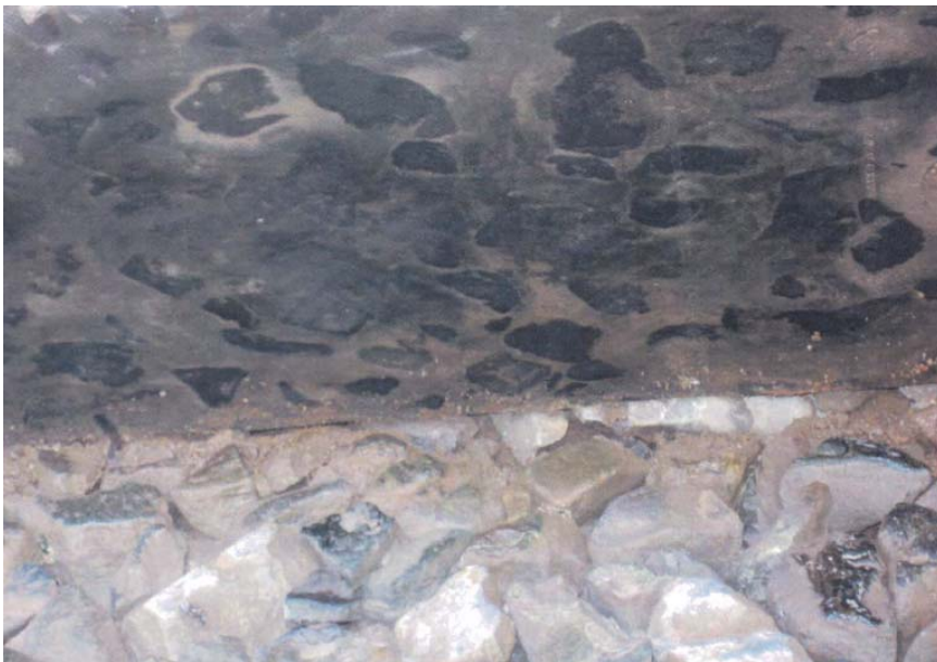
Picture 8: Condition under tie pad
