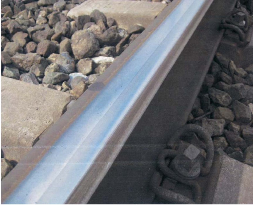
Picture 7: Rail wear
