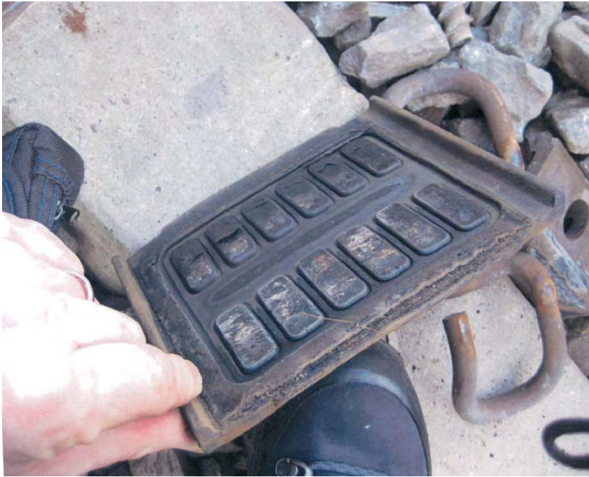
Picture 9: Condition of the rail pads
