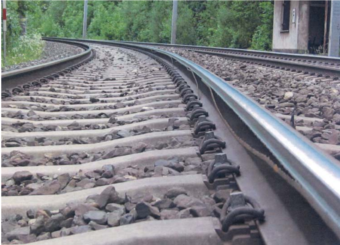
Picture 11: rail wear
