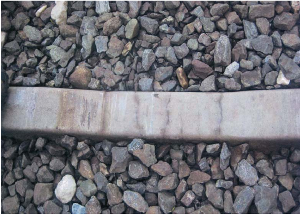
Picture 13: Tie wear
