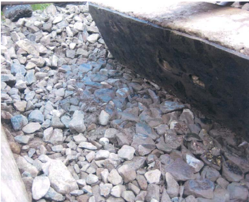
Picture 10: Ballast condition
