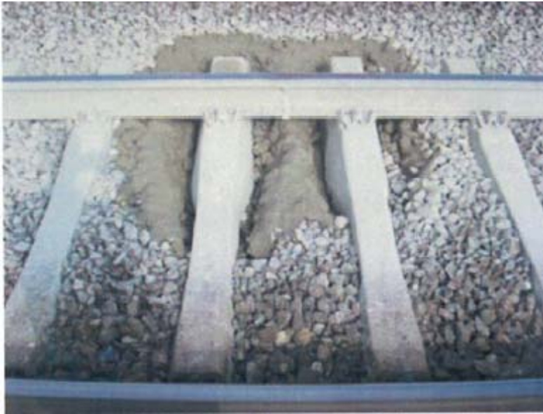
Picture 17: Mud spot due to deferred maintenance of the ballast
