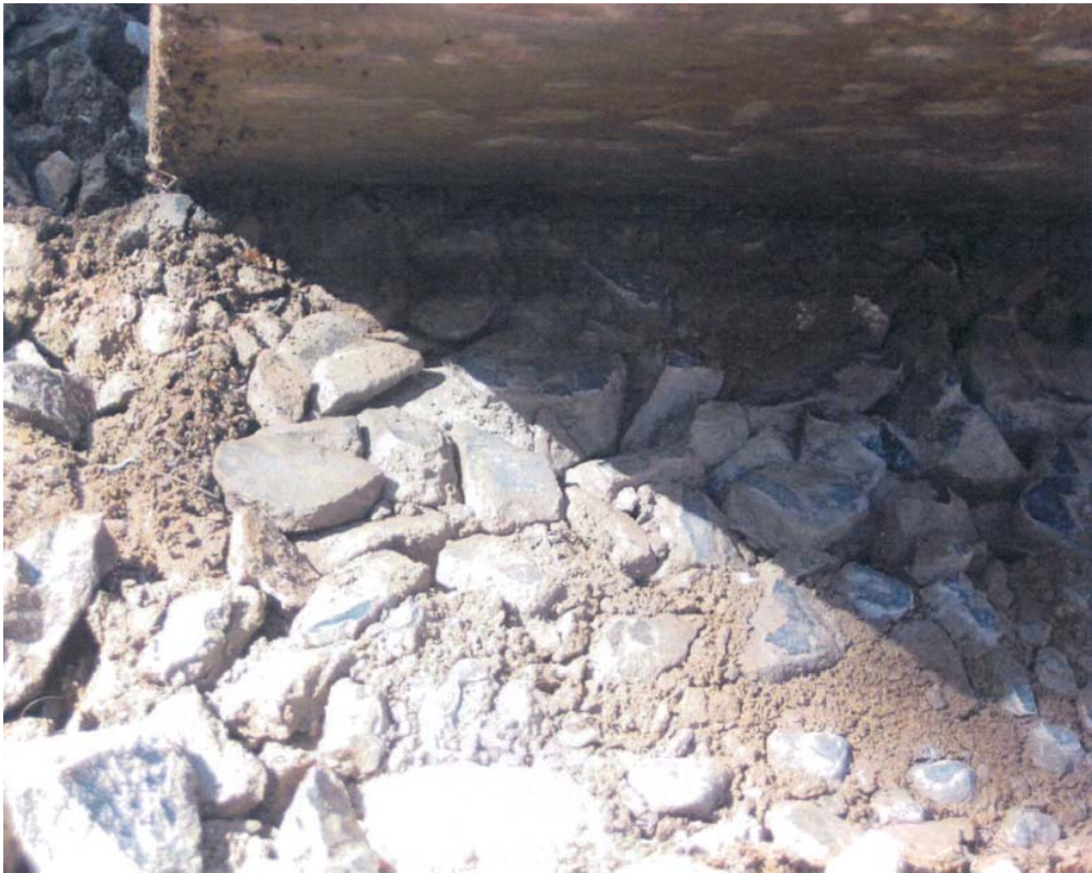
Picture 15: Ballast condition
