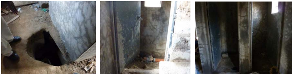
Figure 49 a - c. Construction of a bio-centre a) hole in the concrete slab and the dome, b) toilet, c) showers (Source: Author)
