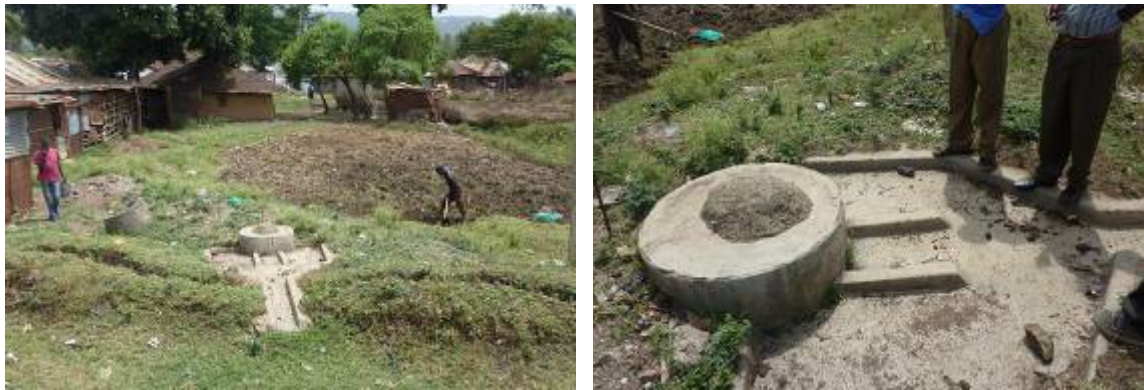
Figure 51 a, b. Abandoned borehole due to contamination by a nearby pit latrine (Source: Author)
