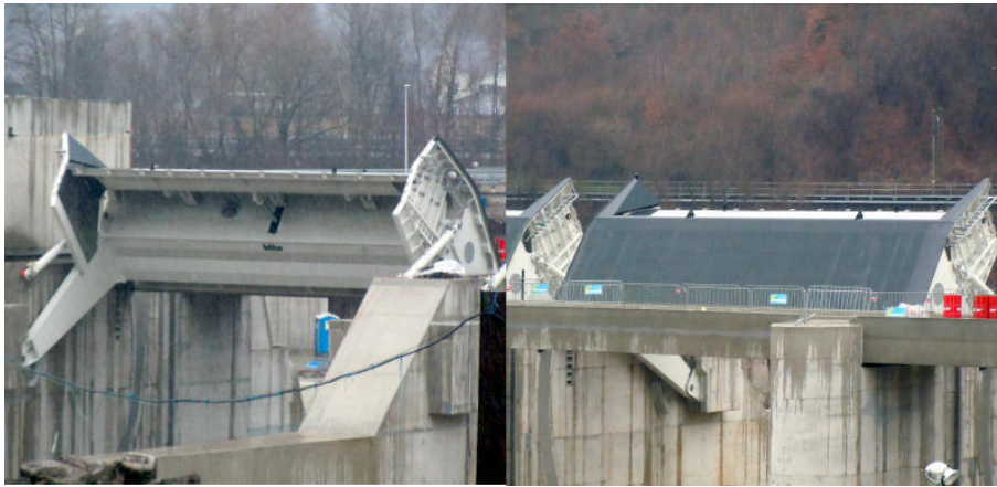
Figure 3-6: Radial gate with fitted flap of the run-off-river plant Rothleiten at the river Mur
