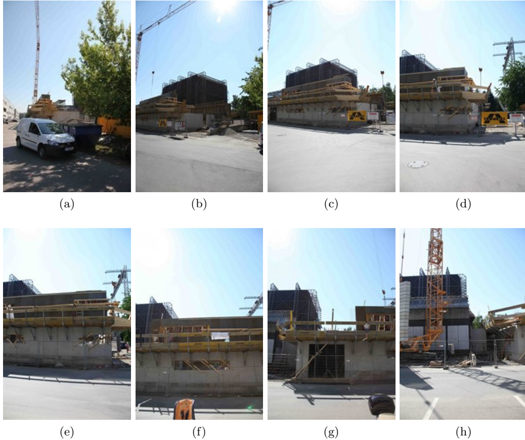
Figure 5.2: Selection of several images from the first dataset temporally ordered. The images were taken from two sides (north and west) of the construction site.
