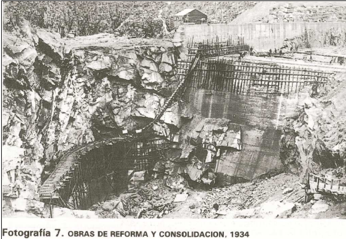
Fig.5 12: Repair works on the spillway in summer of 1934. Construction of a concrete wall at the front slope of the spillway. Looking at the curvature of the wooden balk, the initial shape of the plunge pool can be recognized (Guia tecnica, 1997).
