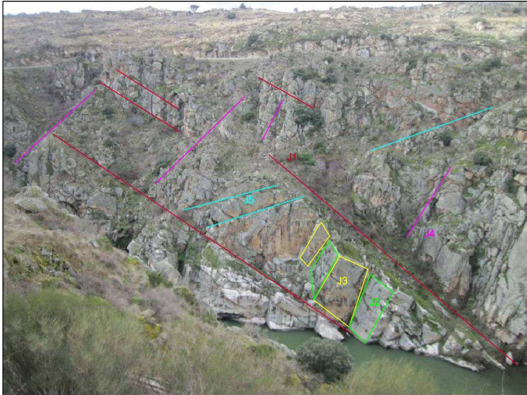
Fig.6 20: View to the right riverbank downstream of the dam, showing the appearance of the rock mass at the Ricobayo dam. Joint patterns of the five joint sets are illustrated. Numbers and colors correspond to the joint orientations in Tab.6.9.
