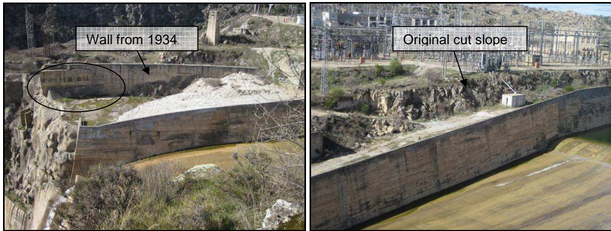
Fig.6 15: View to the right side of the spillway. End of the upper channel. The old wall is still visible in the back and was shifted towards the center of the spillway (left). Cut slope adjacent to the concrete wall of the spillway
