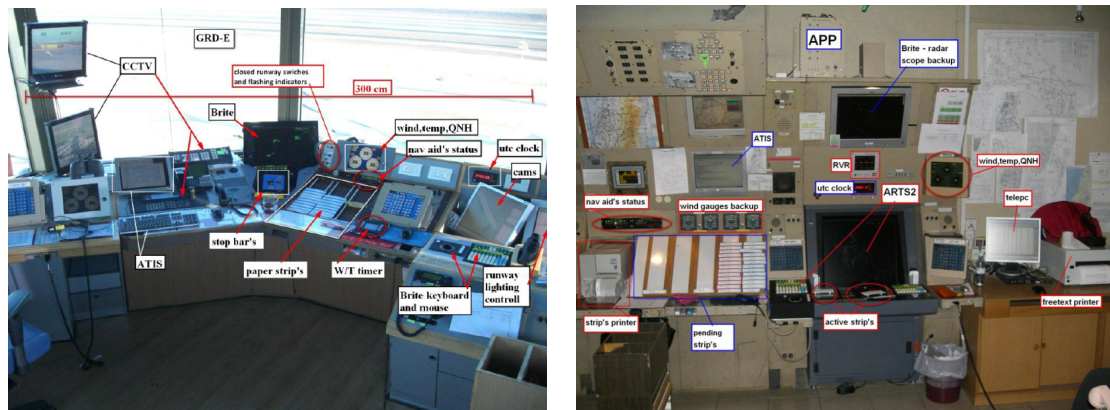
Figure 1.1: These images show the traditional look of an ATCO's working position. We see that the whole working environment is cluttered with a multitude of different systems that seem to be placed wherever some room was left.
