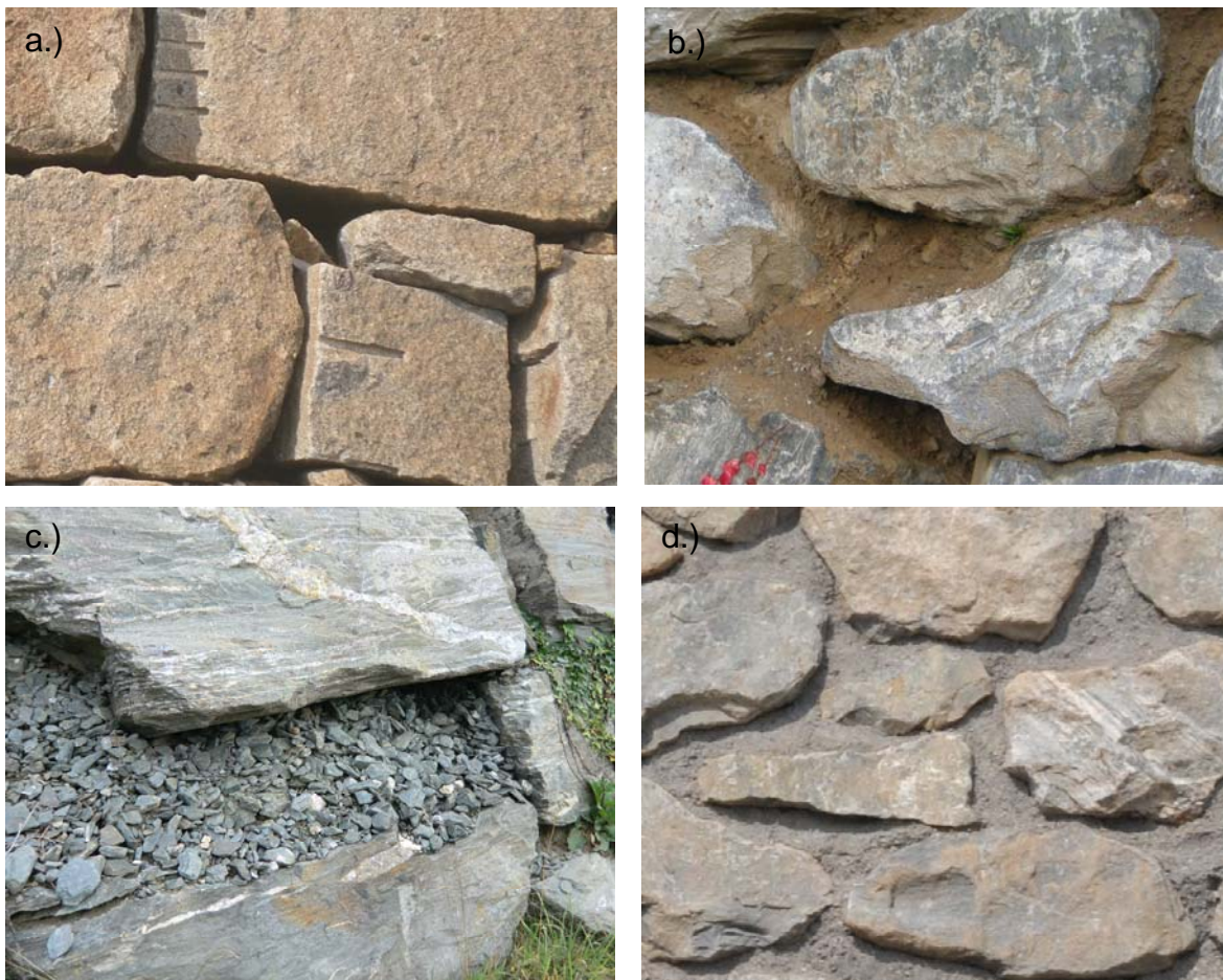
Fig. 6: Different types of chinking a.) no chinking, b.) fine grained material, c.) angular, coarse grained material, d.) mortar
