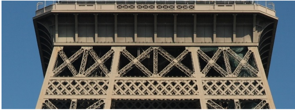
Figure 2.5: A photograph of part of the Eiffel Tower (Released under CC-BY-SA 3.0 by Benh Lieu Song) in which the support grid of one of the platforms of the Eiffel Tower is shown. Note how the grid bars align over the distinct grids.
