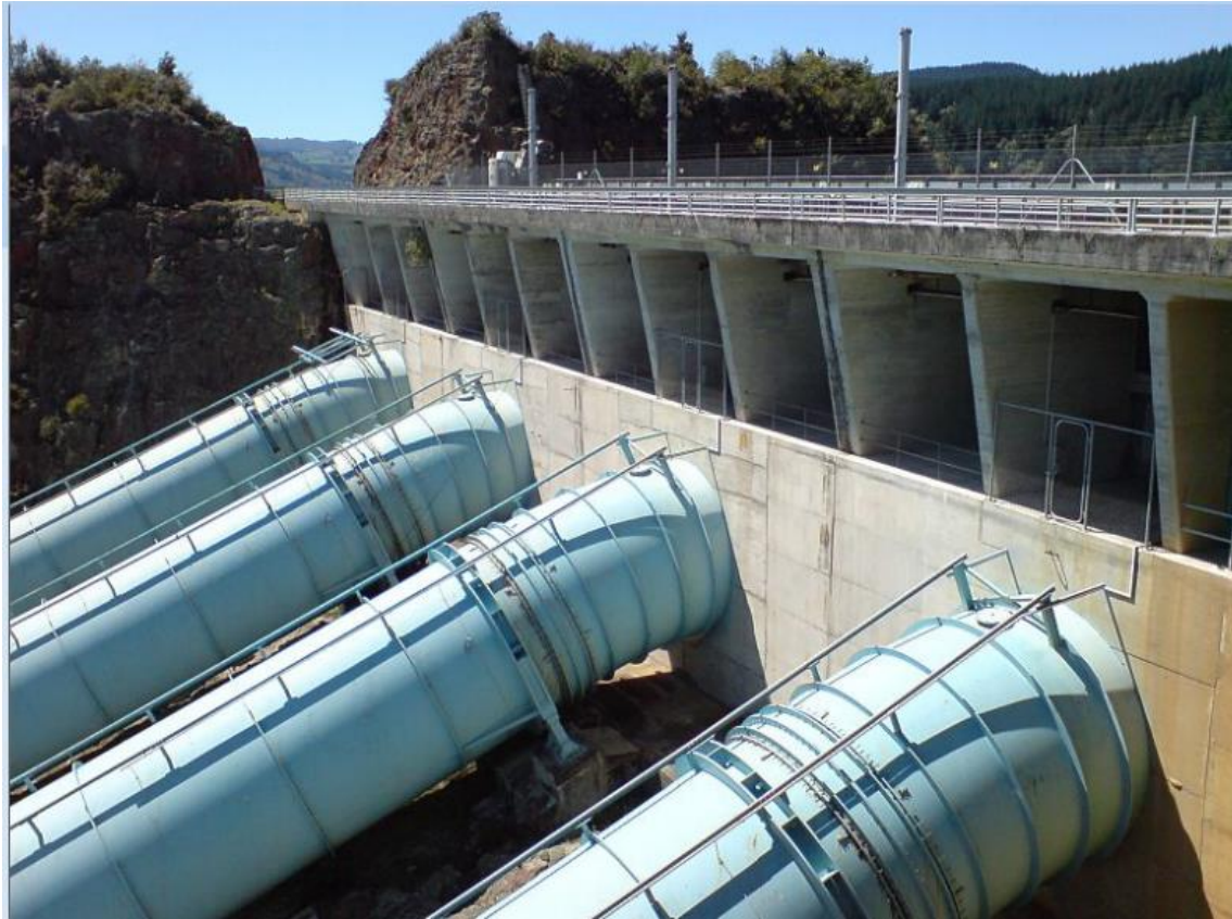
Figure 4: Penstocks, Ohakuri Dam New Zealand [3]
